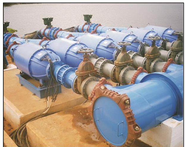
Figure 1 – Amphibious Pumps in Modular System
